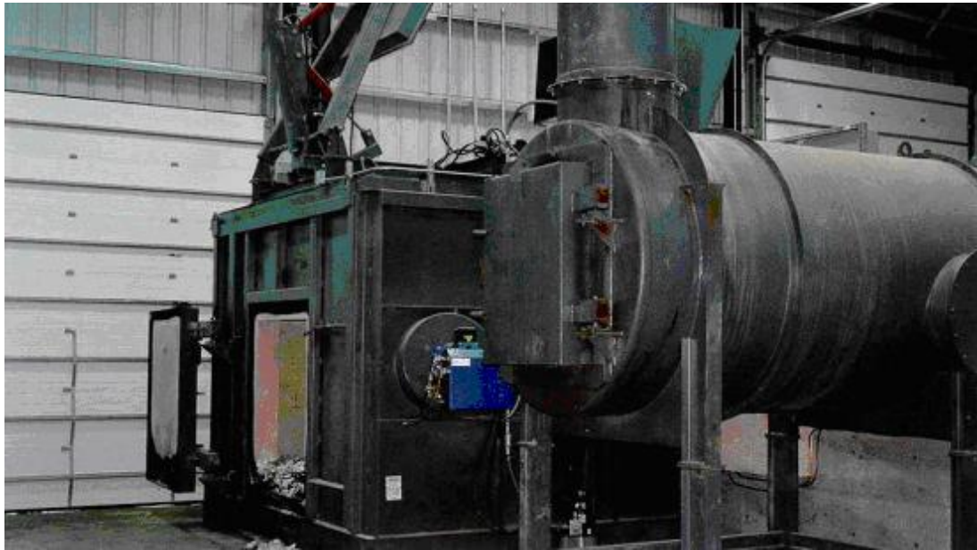
Figure B-7: Egegik Batch Oxidation System.
