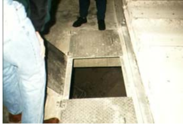
Figure C-9: Ash falls through grate.
