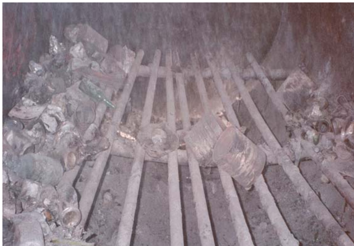
Figure A-10: Note glass at clean-out.
