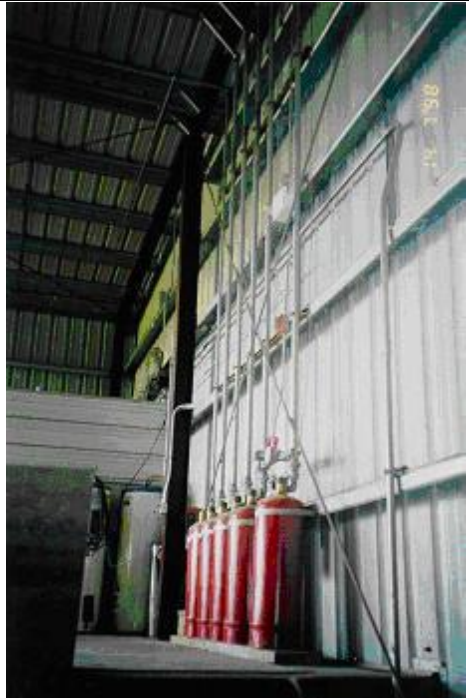
Figure B-6: Fire suppression system in incinerator building.
