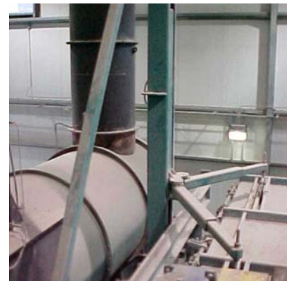
Figure C-7: Secondary chamber (left) and primary chamber (right).
