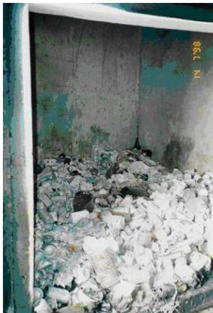
Figure B-4: Ash in primary combustion chamber following burn cycle.
