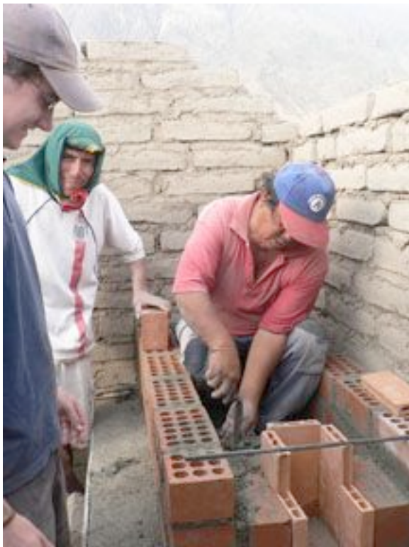
Chris works with Don Norberto and Omar to build the stove in the primary school's comedor .
