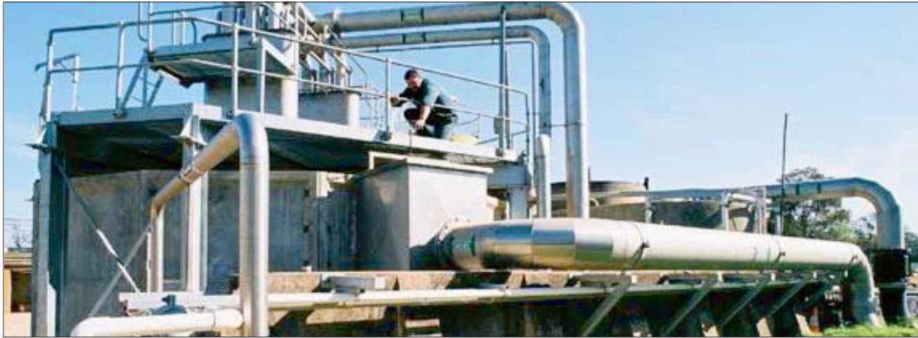
An Environmental Group ozone/GAC water treatment plant that can produce high quality re-usable water from treated sewage.
