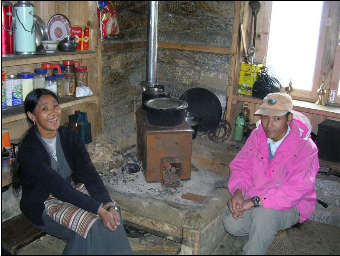
The new stove placed on the open fireplace. Prior to the installation, the lady had a metal rack on which the pots and a kettle were placed. High above the fireplace is a large open hood. The chimney pipe goes into the hood.
