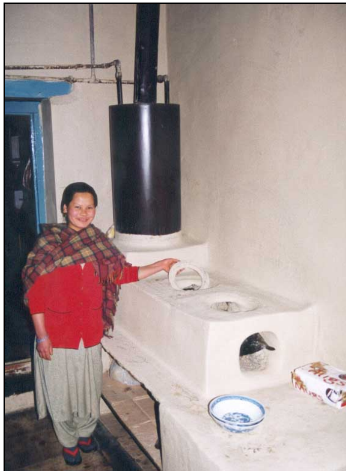
Smoke water heater in a hotel restaurant in Jomsom. On this stove, a mouthpiece and air-intake regulator will improve firewood efficiency. Large mud stoves contribute little to space heating.
