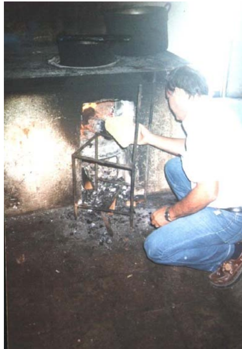
Fig. 9: SFBs feeding in the burning chamber
