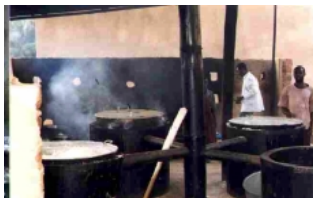
Figure 9: Insufficient chimney capacity causing smoke
