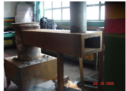
Large Modified Heat Exchanger
