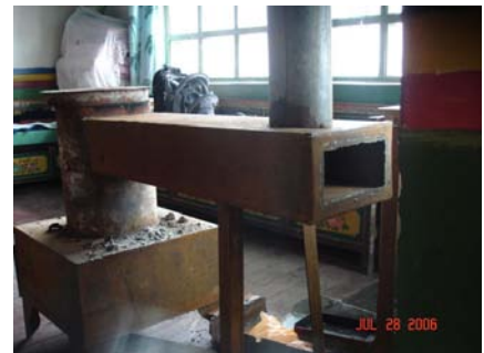
Large Modified Heat Exchanger
