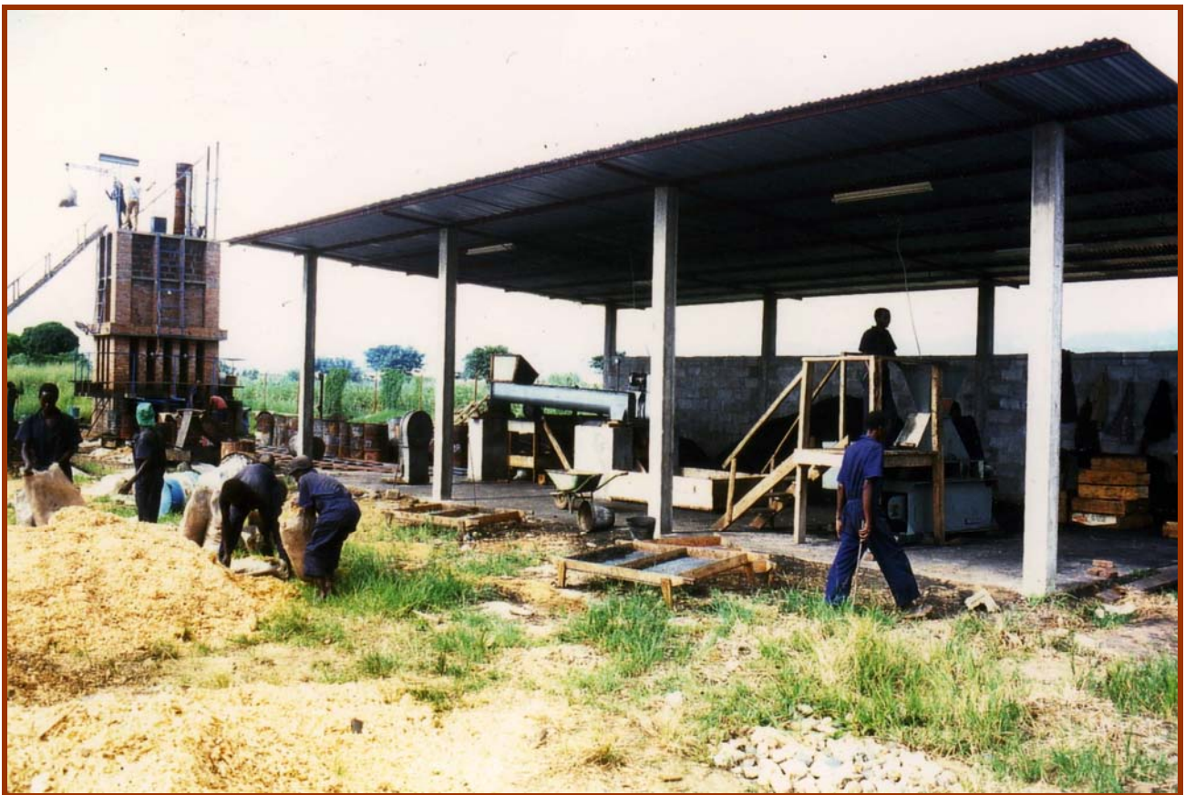
Photo 2: production hangar, roller press (with a staircase for top loading) on the right side
