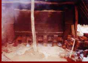
Using Paddy Husk to burn bricks in an Improved kiln in Anuradhapura District
