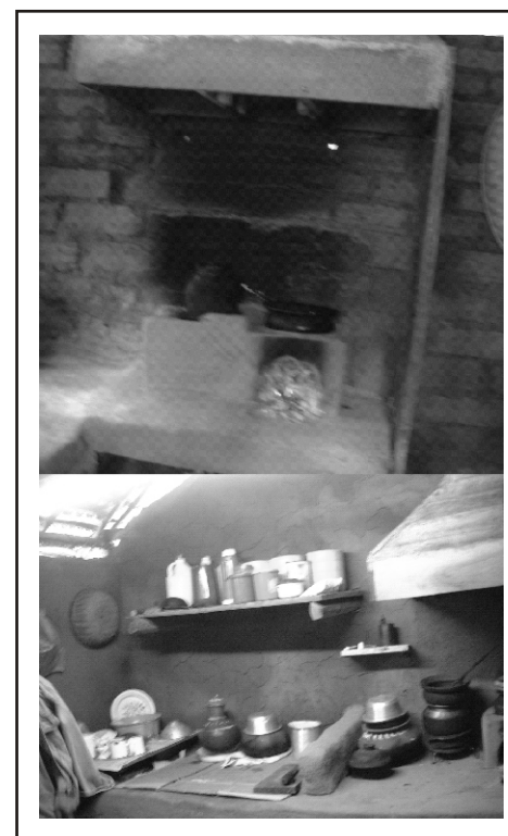
Chimney hood (wood and mud) installation and introduction of racks, as part of household kitchen
